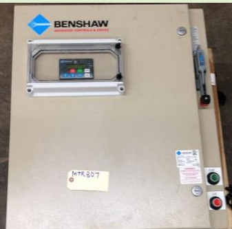
Pump Motor Starters
